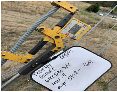
Anchor A Guy Level 1
