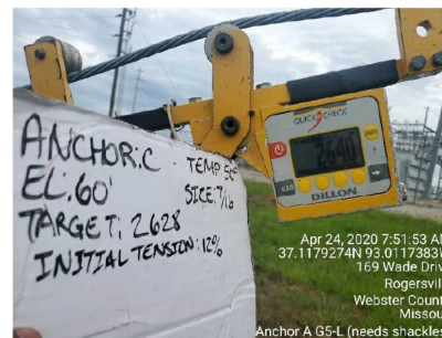
Anchor A Guy Level 2
